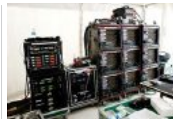
Racked equipment from L-Acoustics, DiGiCo and Sennheiser
